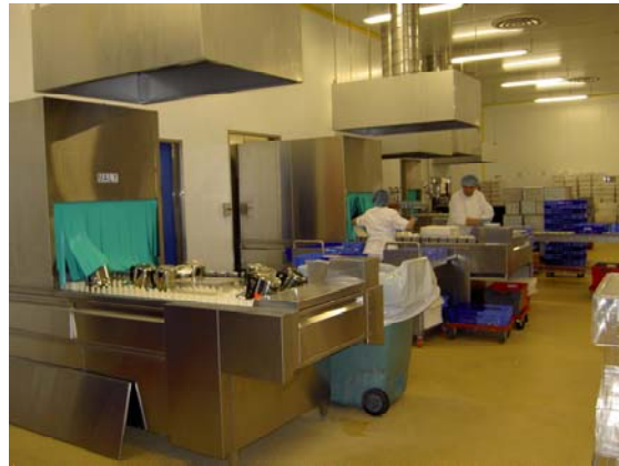
Commercial dishwashing lane
